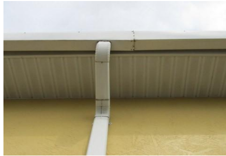
Pictures of current gutter system with deficiencies
