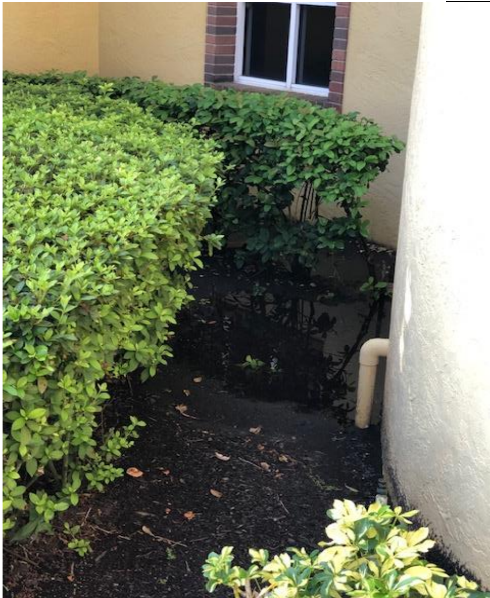
Pooling water in area recommended to install new gutter system
