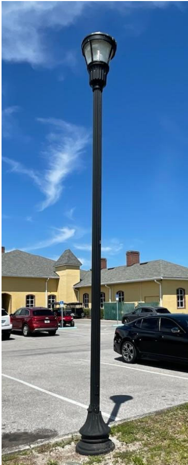
Existing Salem Post Top Fixture and Franklin Pole
